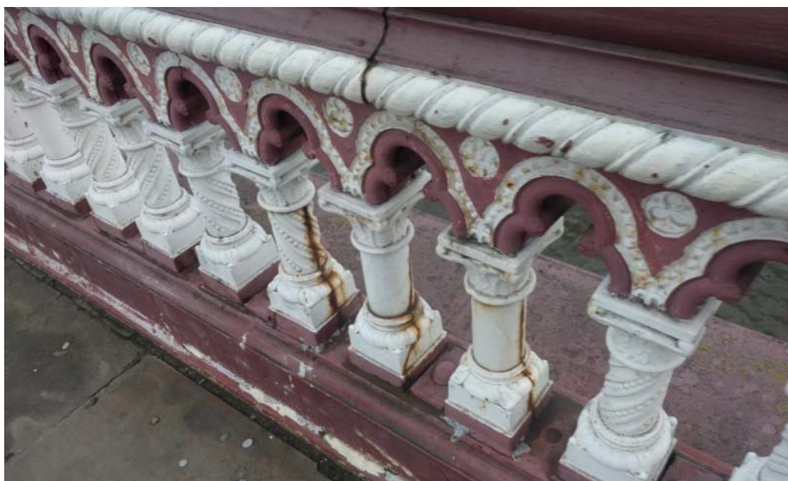
Figure 5. Example of the rusting staining of the vertical casting joints
