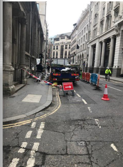
Pavement narrowed due to scaffolding and cyclists
