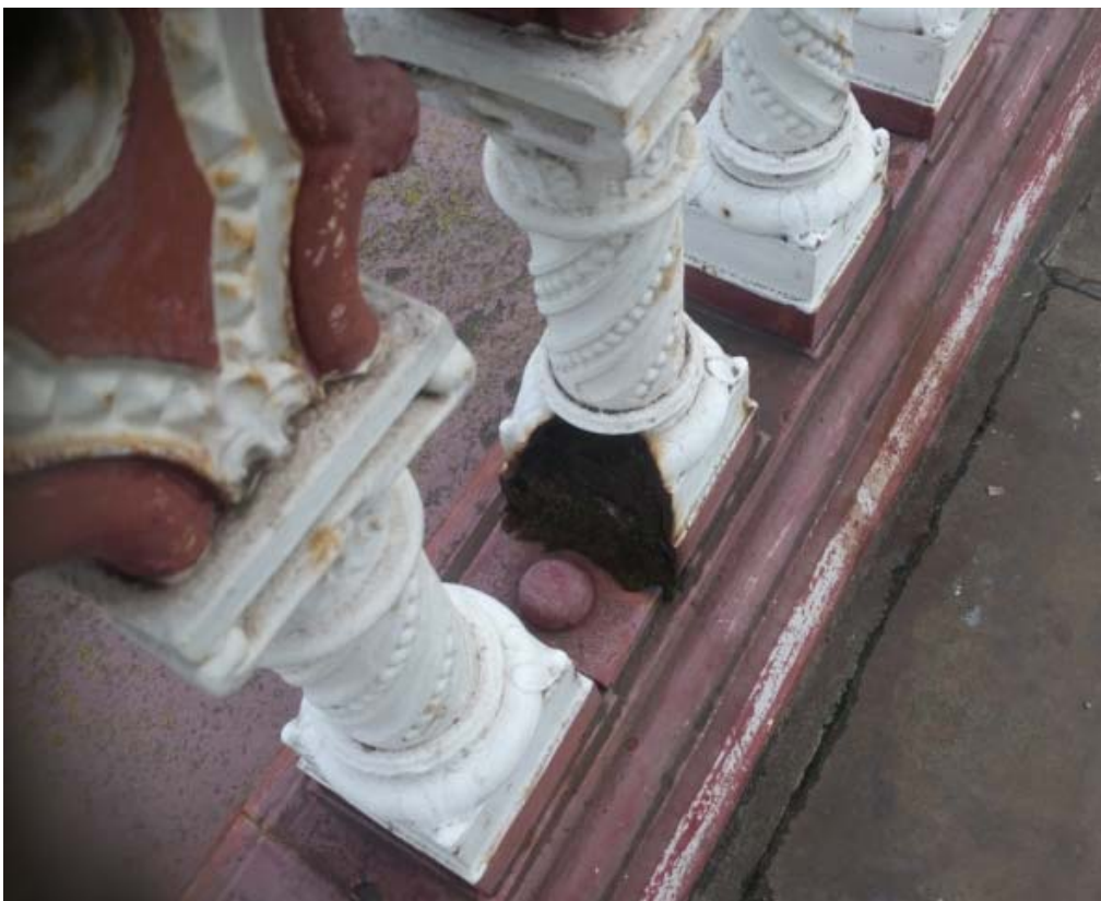
Figure 7. An example of section loss at the base of the baluster
