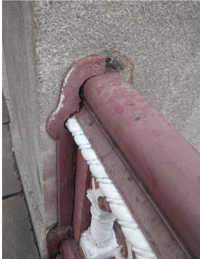
Figure 6. A missing plate connecting the parapet to the pier
