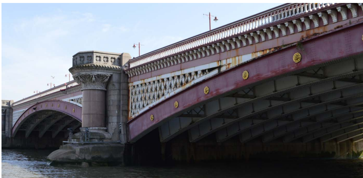
Figure 157. Current rust staining on the bridge
