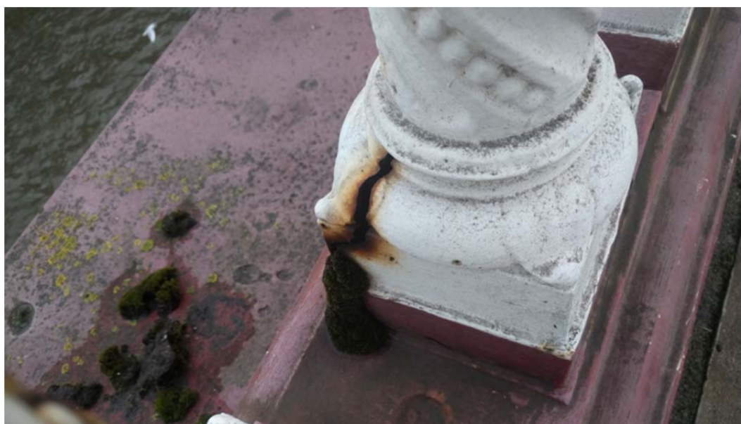
Figure 4. Example of large crack in the corner of baluster base that is required to be filled with epoxy filler.
